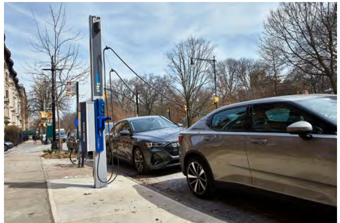
Figure 11. New York City worked with local utility Con Edison and national charging operator FLO to create 100 on-street charging stations in the city (FLO)
