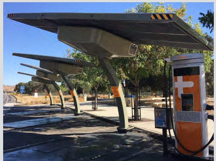
Figure 4. Solar-powered Level 3 fast charger at the Camp Roberts rest area along US 101 in California (Mavila97/Wikimedia (CC BY-SA 4.0))
