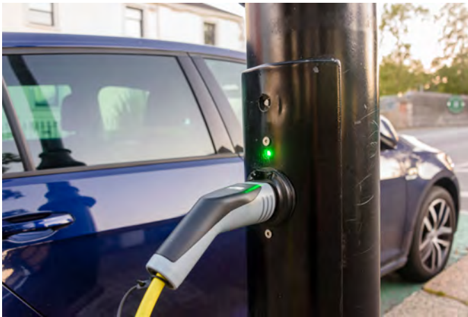
Figure 12. Cities such as Seattle are beginning to install EV charging stations attached to utility poles (Stephen Barnes/iStock/Getty Images Plus)
